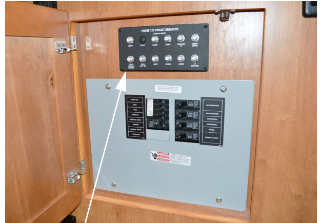
House 12-Volt Circuit Breakers
